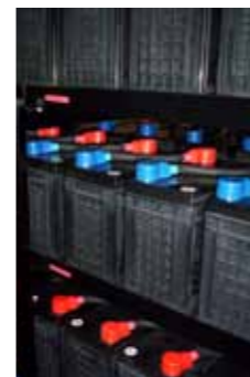
BTX-LS VRLA Batteries
